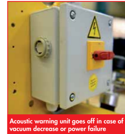
Main switch surveillance by vacuum switch in distribution line
